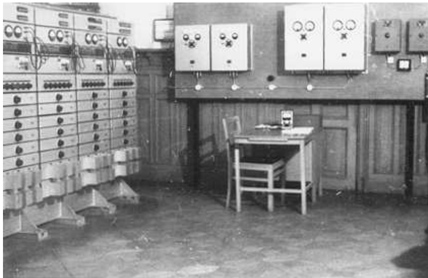
Figure7. Another view from the rack room.
